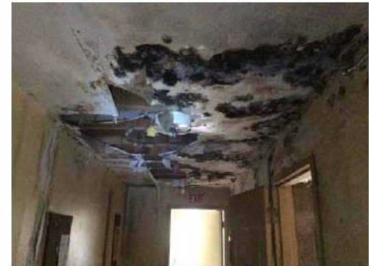
PHOTO #36: WATER DAMAGE, CENTRAL HALLWAY
