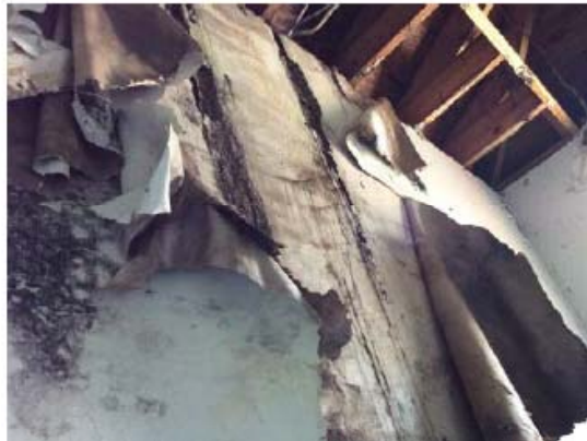
PHOTO #39: WATER DAMAGE
