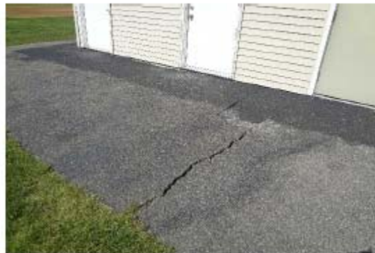
#6: PEDESTRIAN PAVEMENT, SIDEWALK, CRACKING
