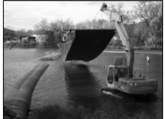
Engineering Enterprises Inc., of Sugar Grove, installs a cofferdam for the city's water treatment project. The temporary fixture was used for one week.
