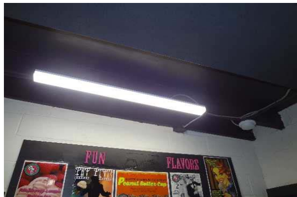
#34: LIGHTING SYSTEM, INTERIOR - FOXY'S ICE CREAM
