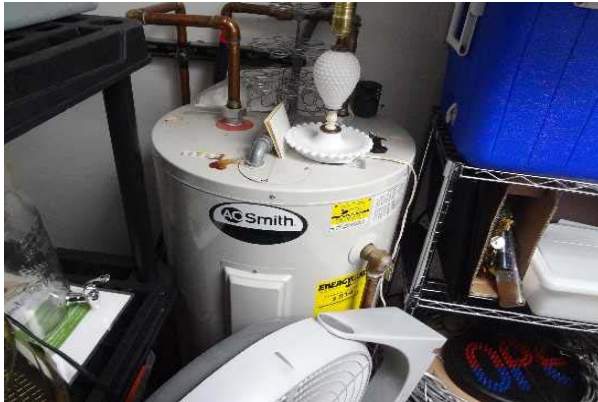
#25: WATER HEATER, ELECTRIC - GINGER + SOUL
