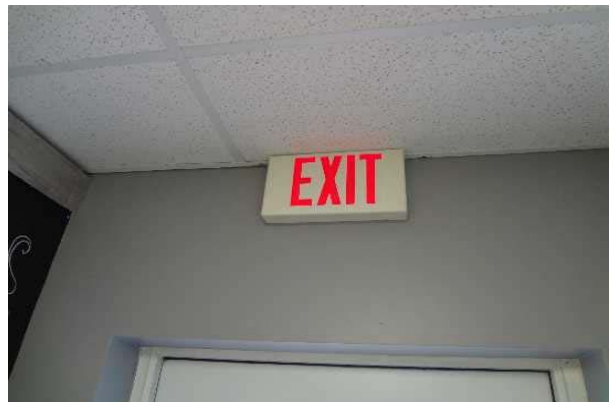
#42: EXIT LIGHTING FIXTURE
