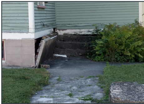
Image 6: Dangerous Settling around the Foundation
