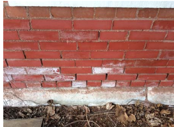
PHOTO #16: EFFLORESCENCE AND MISSING MORTAR
