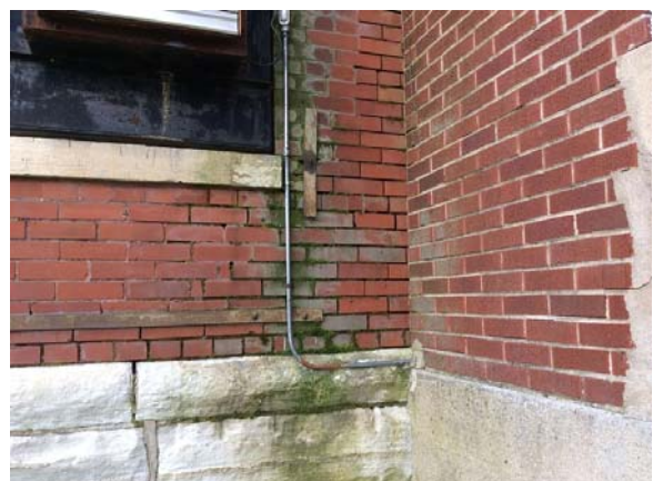
PHOTO #12: MISSING MORTAR
