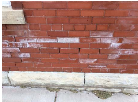
PHOTO #10: EFFLORESCENCE AND DETERIORATED MORTAR
