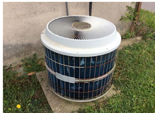
PHOTO #18: CONDENSING UNIT
