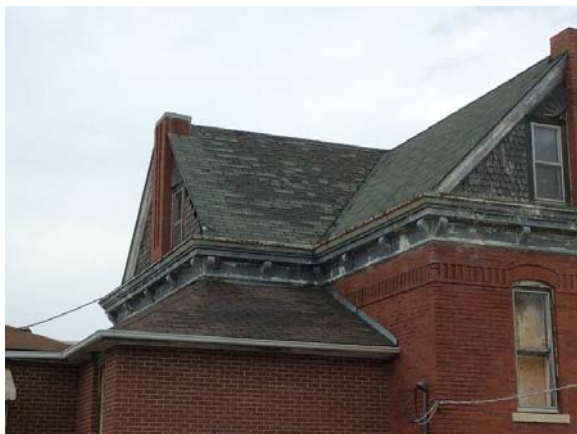
PHOTO #9: ASPHALT SHINGLE ROOF, DETERIORATING
