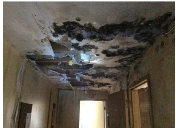
PHOTO #36: WATER DAMAGE, CENTRAL HALLWAY
