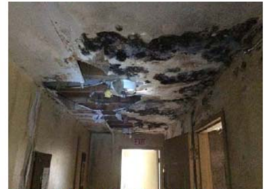
PHOTO #36: WATER DAMAGE, CENTRAL HALLWAY
