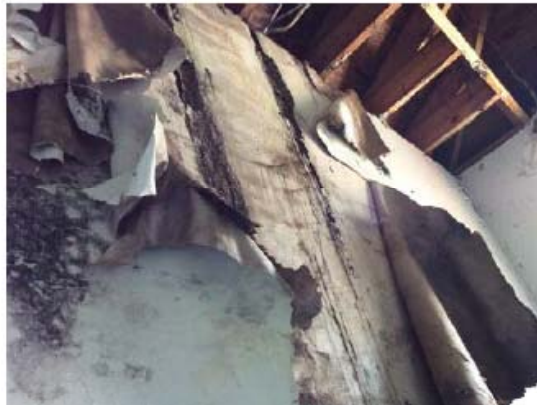
PHOTO #39: WATER DAMAGE
