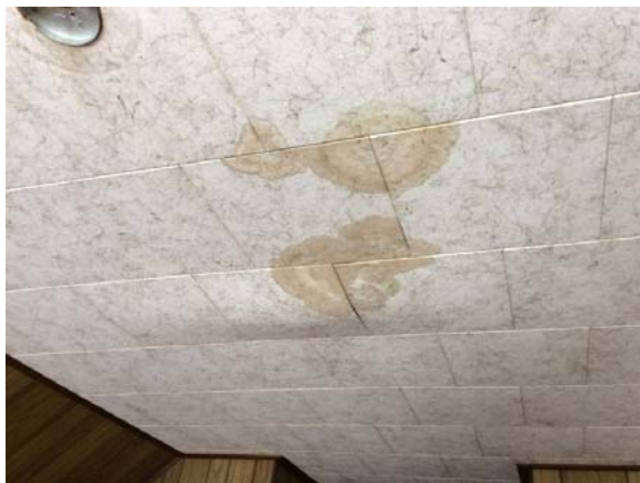
PHOTO #57: WATER DAMAGE, THIRD FLOOR
