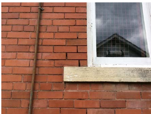
PHOTO #11: MISSING MORTAR
