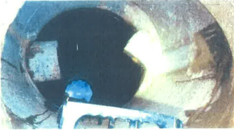
Restrictor Structure 292 with 4" restrictor on inlet side.
